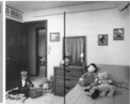
Long, narrow cove radiant heater is located on wall up near ceiling
